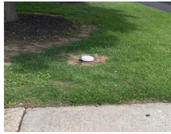
Example of a Maple Shade Clean Out
