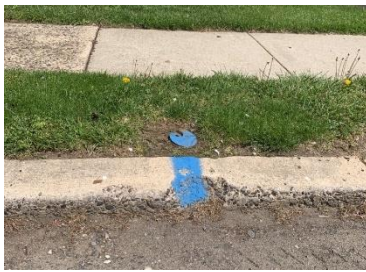
Example of a Maple Shade Curb Stop
